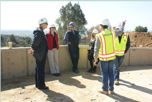
Construction management team leads tour for Cheryl Marshall, Rebecca Warren-Marlatt and Larry Cook.
