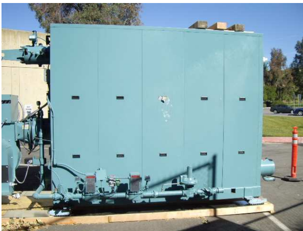
Boiler is ready to be installed at the Central Plant as part of Package #2/3/4
